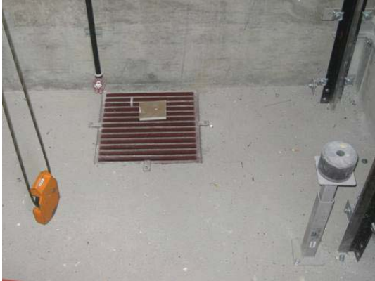
Sump with cover
