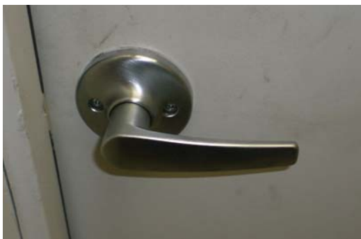
Door handle inside machine room
