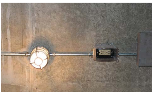
Pit light and receptacle
