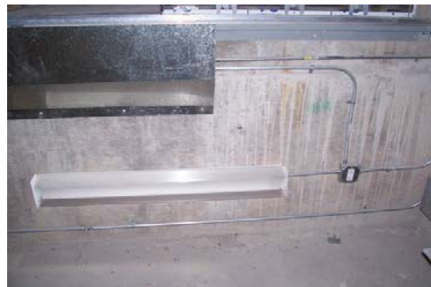
Fluorescent pit light
