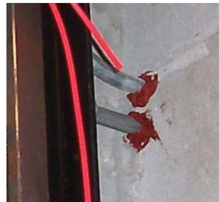
Hoistway penetrations filled with fire caulking to maintain fire rating
