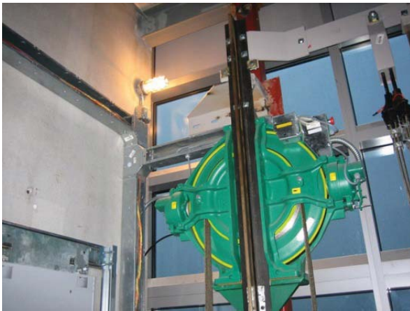
Machine space lighting at top of hoistway
