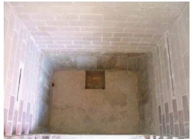
Clean dry pit with sump
