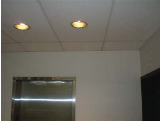
Finished lobby ceiling light
