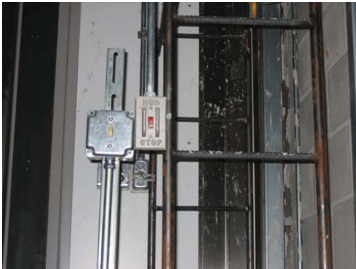
Pit ladder, light switch, stop switch
