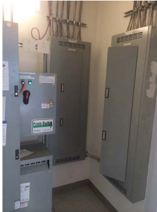
Shunt Trip Breaker
