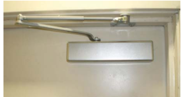
Closer on machine room door
