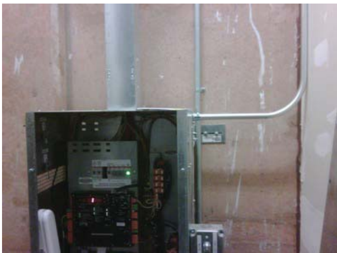
Phone line piping to controller
