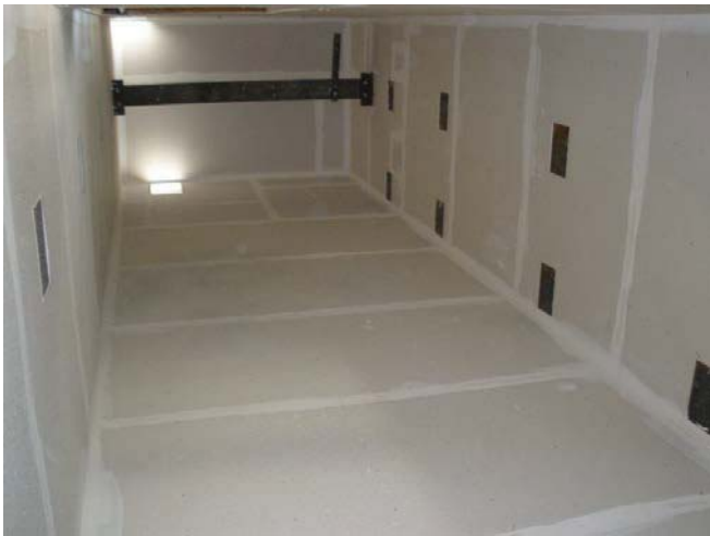
Steel plate attachments in hoistway
