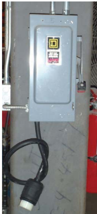
Temporary power for Tirak hoist
