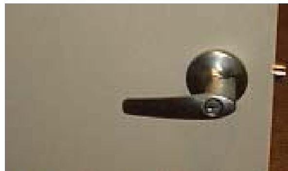
Door handle outside machine room
