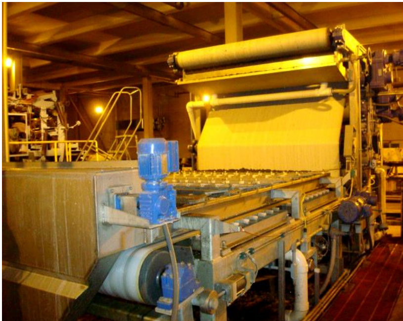
Two-Meter Belt Filter Press
