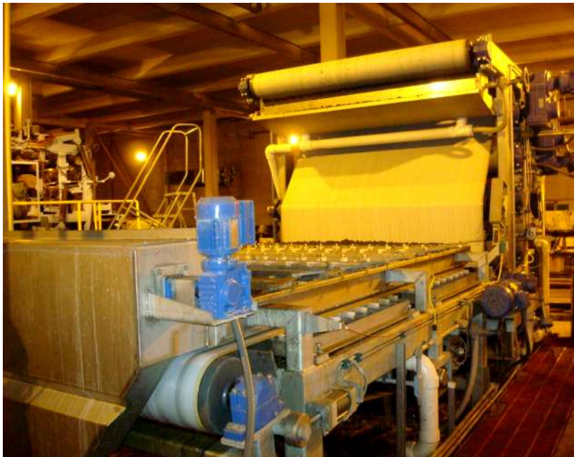
Two-Meter Belt Filter Press
